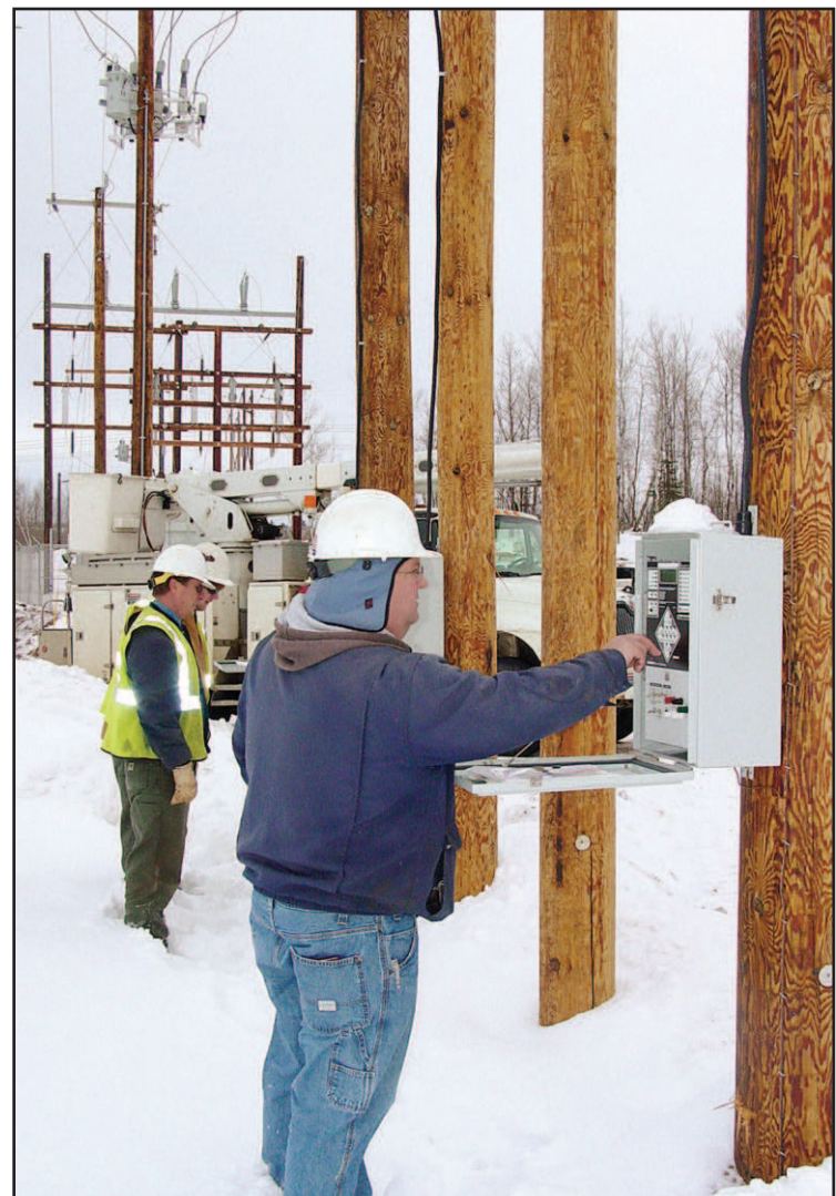
NATHAN BERGSTEDT/GRAND RAPIDS HERALD REVIEW Lake Country Power's engineers and line crews building the substation that exclusively serves Magnetation.
