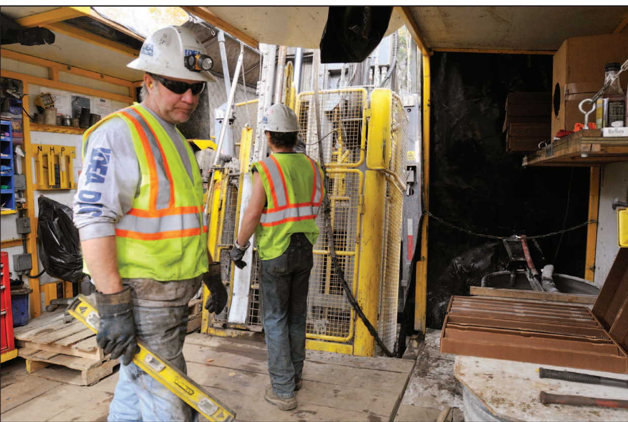
Bruce Ziminske and Jim Snodgrass keep an eye on drill operations as they bore through the last 11 feet of a test hole.
