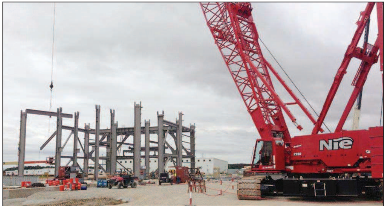
Grand Rapids-based Northern Industrial Erectors (NIE) began erecting the induration building (which will house the furnace) at the discharge end in mid-September and will continue to work toward the feed end of Magnetation LLC's new pellet plant in Reynolds, Ind. NIE was also awarded other projects within the $350 million project.
