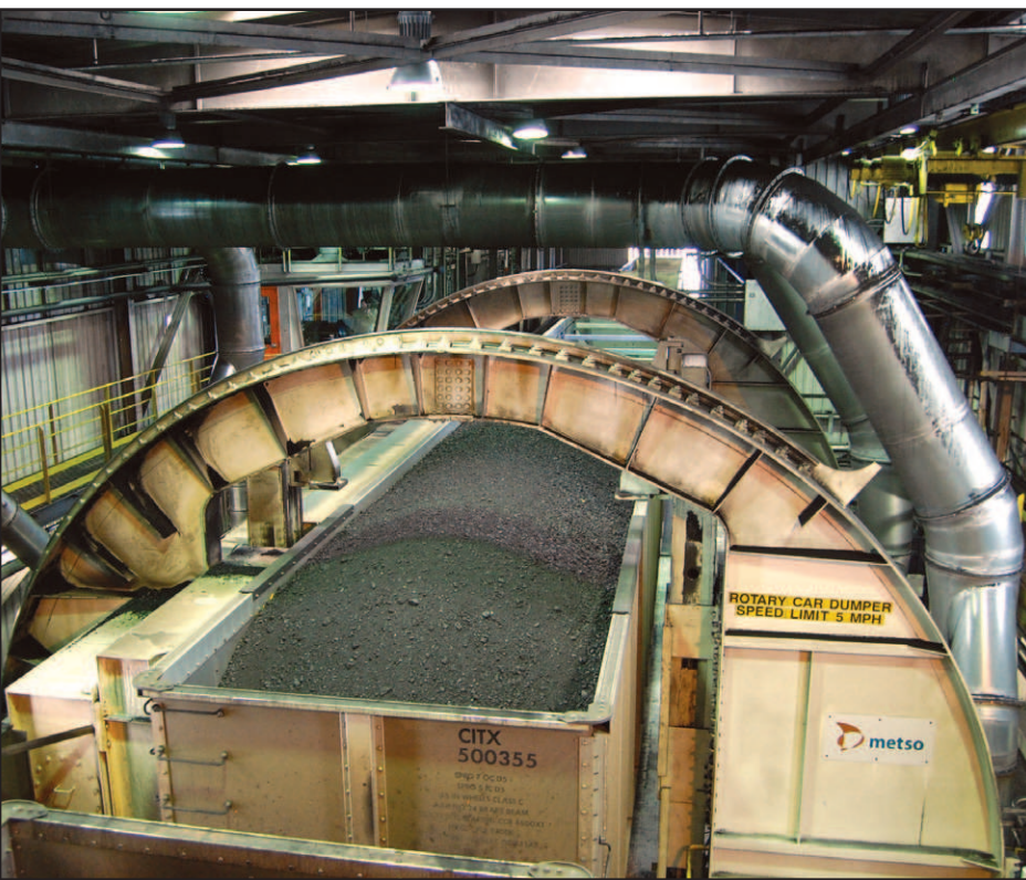
A coal car is moved into place before it is rotated and dumped. The coal falls to a conveyer belt below and is then moved to the Boswell Energy Center's coal stockpile.
