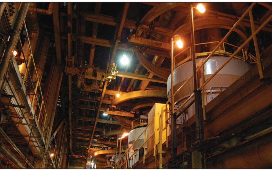
Coal pulverizing equipment at Unit No. 4 at Minnesota Boswell Energy Center in Cohasset. The coal is pulverized into a fine dust, which allows for optimal combustion, before it is injected into the boiler. Optimal combustion is part of the equation for the most efficient transfer of energy from coal to flame to water to steam to electricity, according to a spokesman from Minnesota Power.
